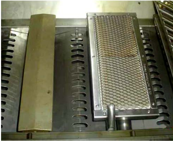
One infrared burner installed
